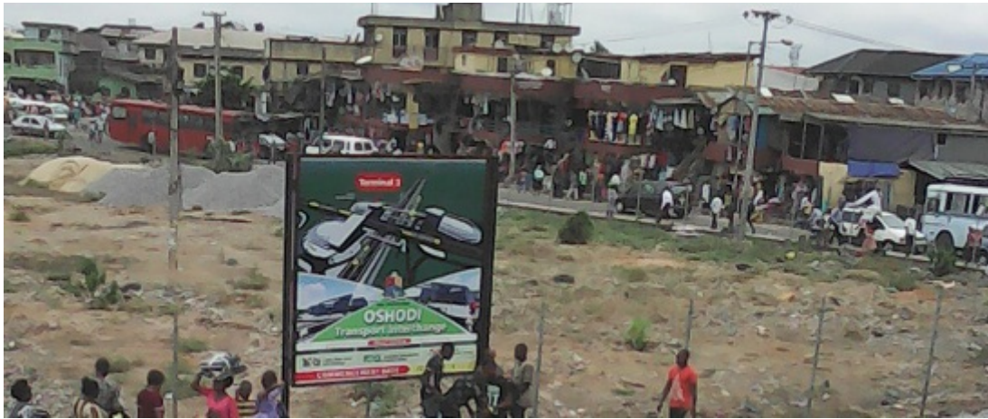
The demolished Owonifari Market, Oshodi, to make way for the 'Oshodi Transport Interchange' (FIWON, August 2016).
