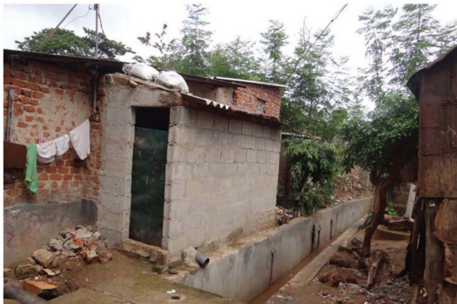
Drainage Construction in Shantipally, Bhubaneswar, Odisha, India © Janhavi Dave, HomeNet South Asia
